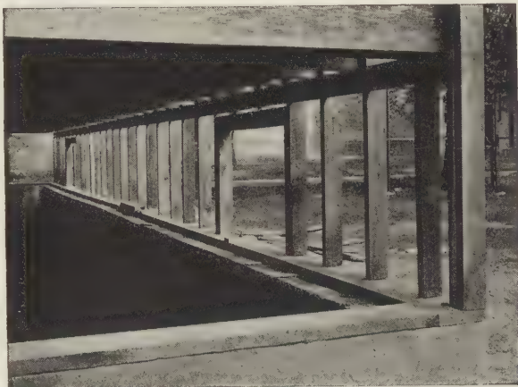
FIG. 28.—Concrete basement wall under residence showing method of anchoring wall plates to wall.
